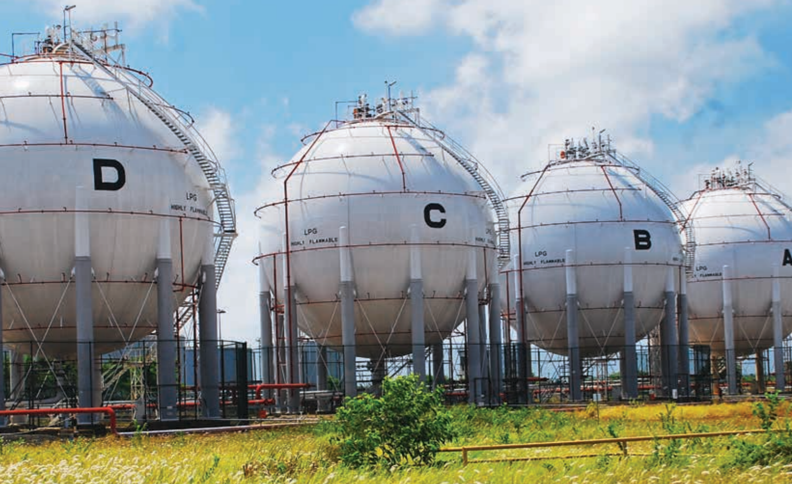
LPG Storage Tanks for Shell Terminal Lanka
